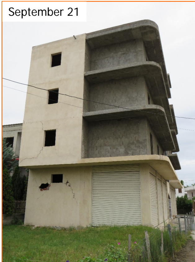
Effect of the vertical component of the earthquake ground motion in combination with the horizontal one on brick walls on an RC cantilever.
