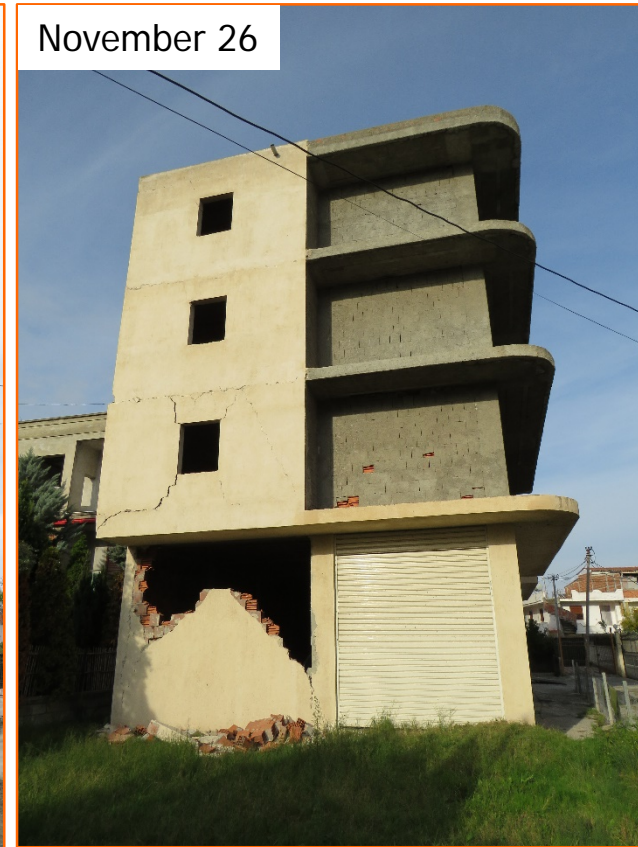
Partial collapse of the brick wall of the ground floor and light cracks.
