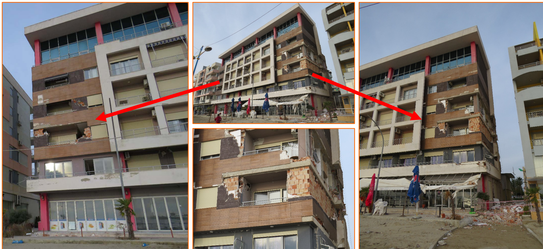
Exterior non-structural walls made of hollow clay bricks outside the reinforced concrete frame suffered damage
