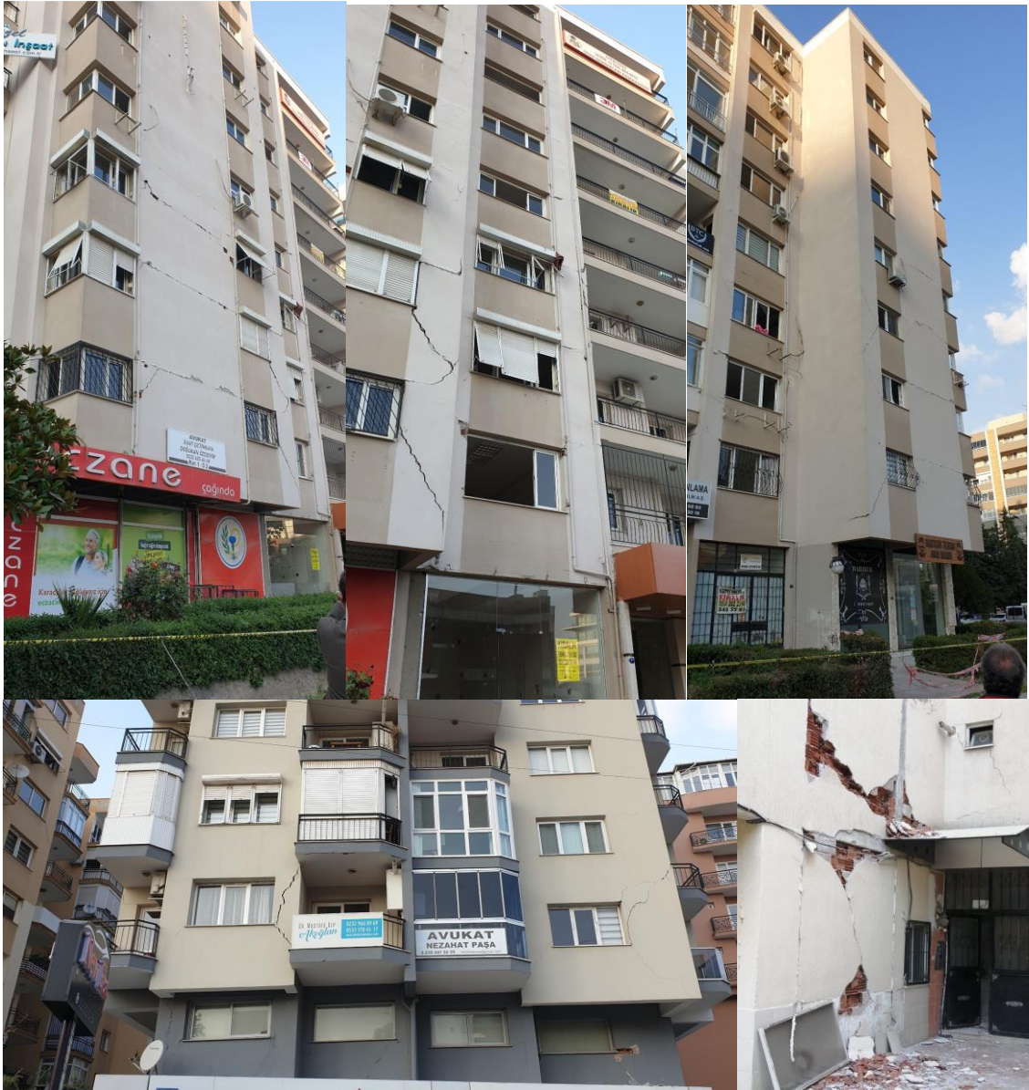
Figure 5.4 Infill wall damages.
