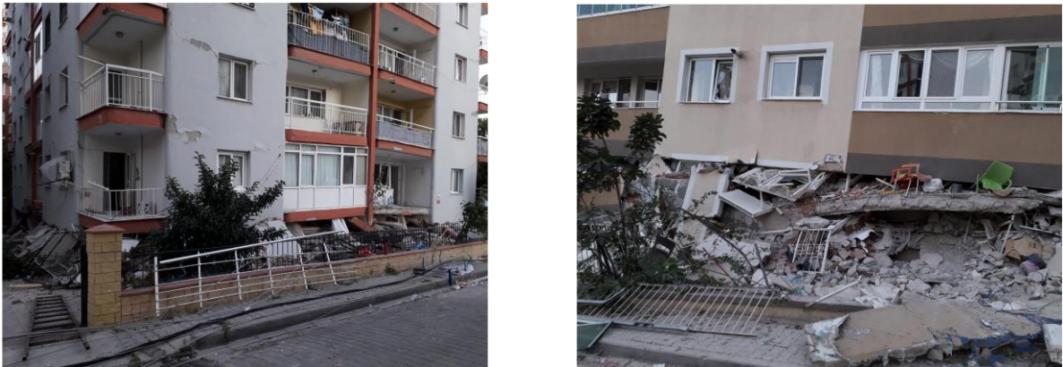
Figure 5.1 Heavily damaged buildings as a result of soft story collapse
