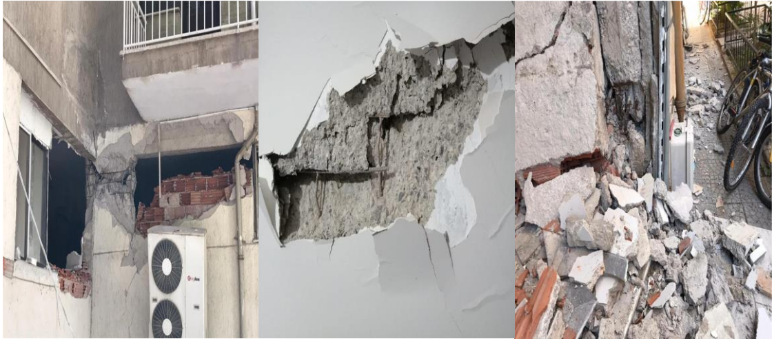
Figure 5.2 Damage due to improper detailing of reinforcement.
