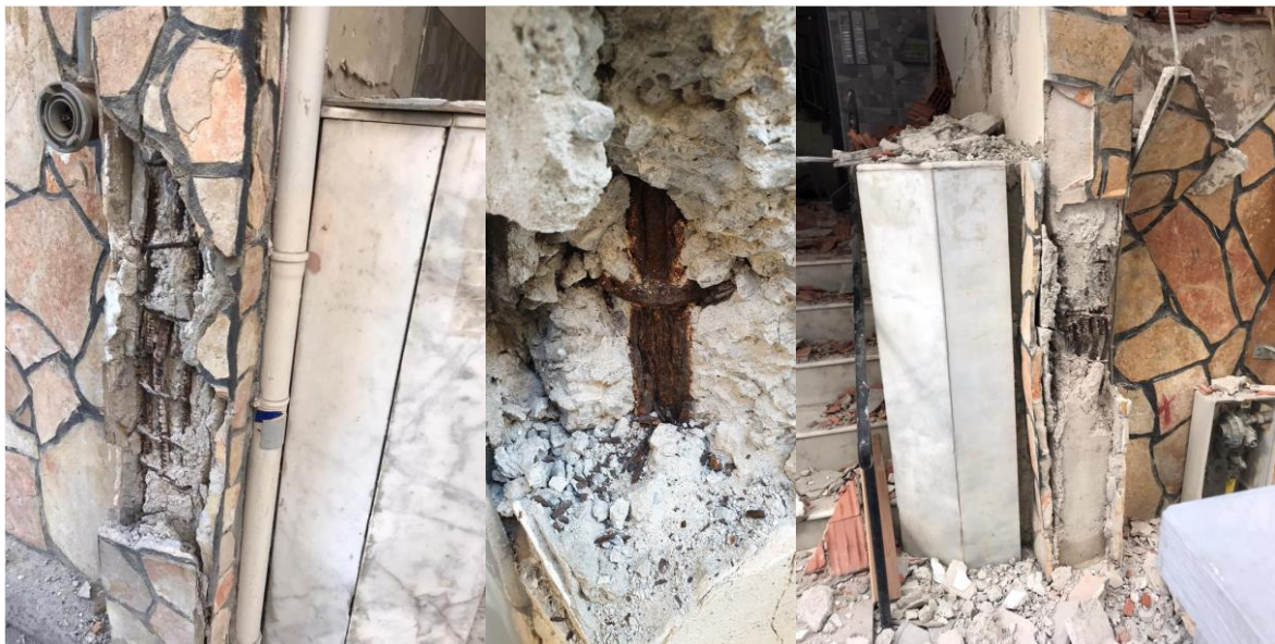
Figure 5.3 Corroded reinforcements and inadequate confinement.
