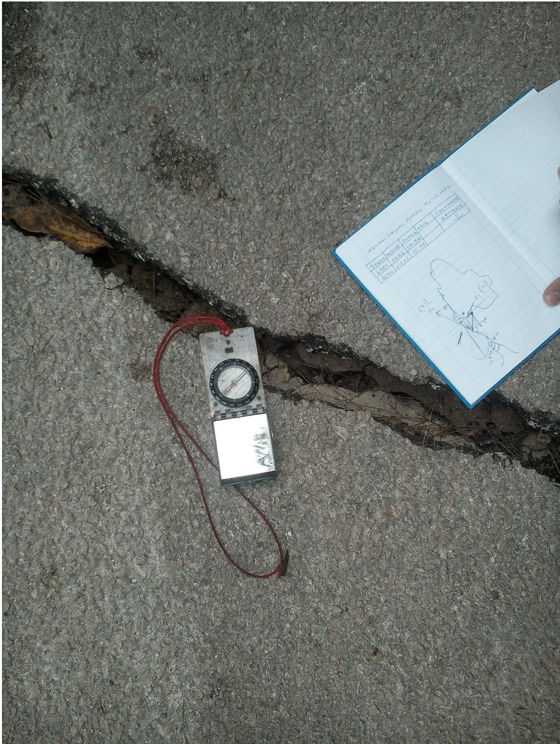
Figure A10 Field photo of 7cm wide tensional crack at Dragano village. Extension azimuth is N130°E. Nadir view. Date photo was taken 22 Nov. 2015.
