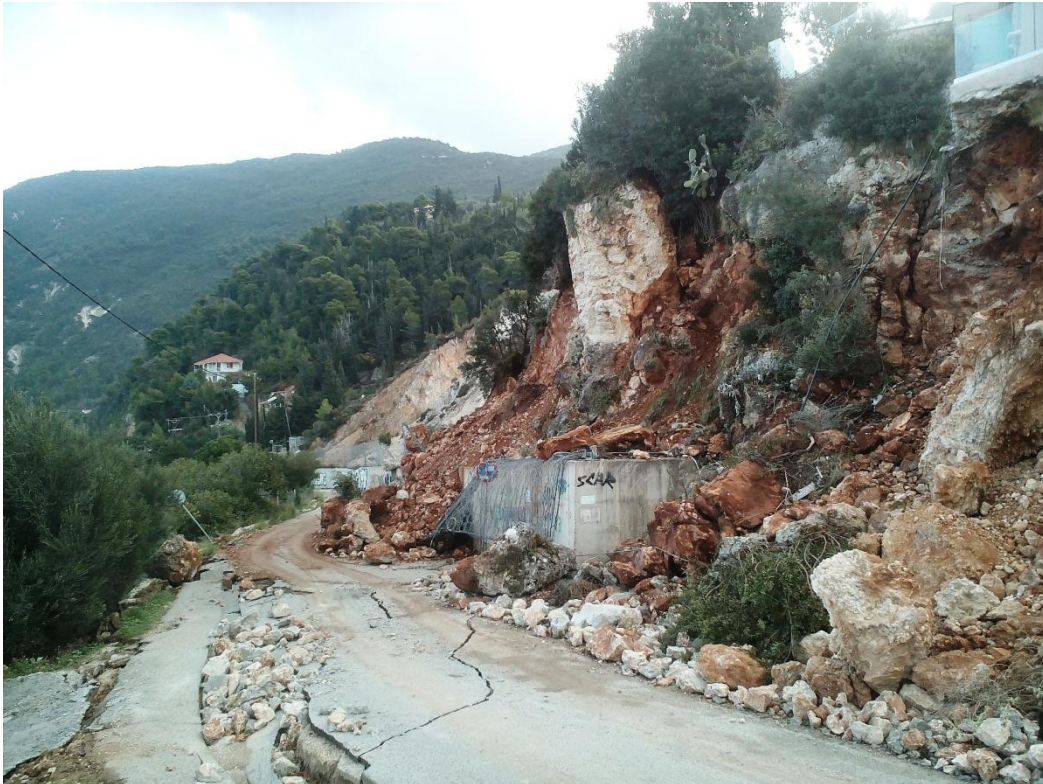
Figure A9 Field photo of landslide at Agios Nikitas village. View to the north. Date photo was taken 22 Nov. 2015.
