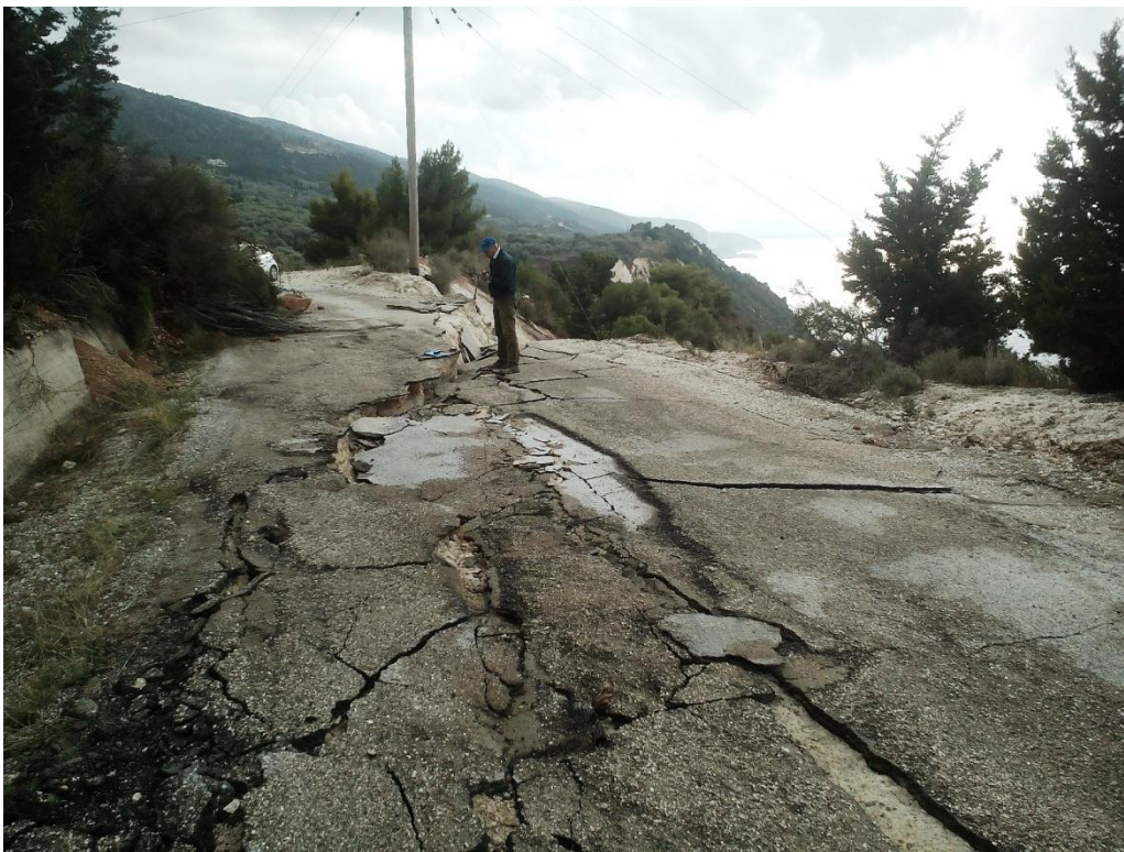
Figure A7 Field photo of damaged road due to landslide at Platys Gialos beach. View to the south. Date photo was taken 21 Nov. 2015.
