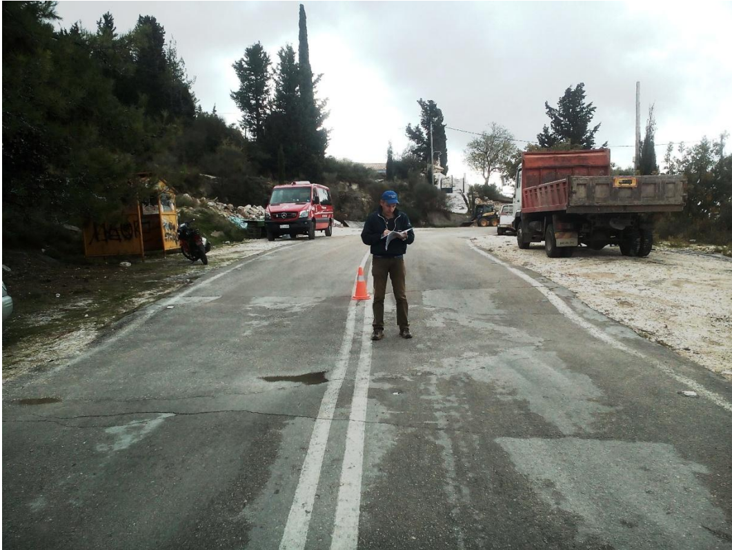
Figure A6 Field photo of damaged road at the entrance of Athani village. View to the south. Date photo was taken 21 Nov. 2015.
