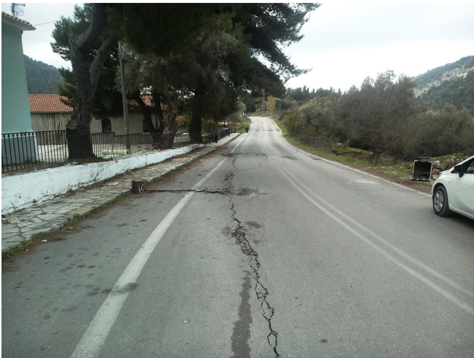
Figure A2 . Field photo of asphalt cracks along the road between Dragano and Athani villages. View to the south. Date photo was taken 20 Nov. 2015.
