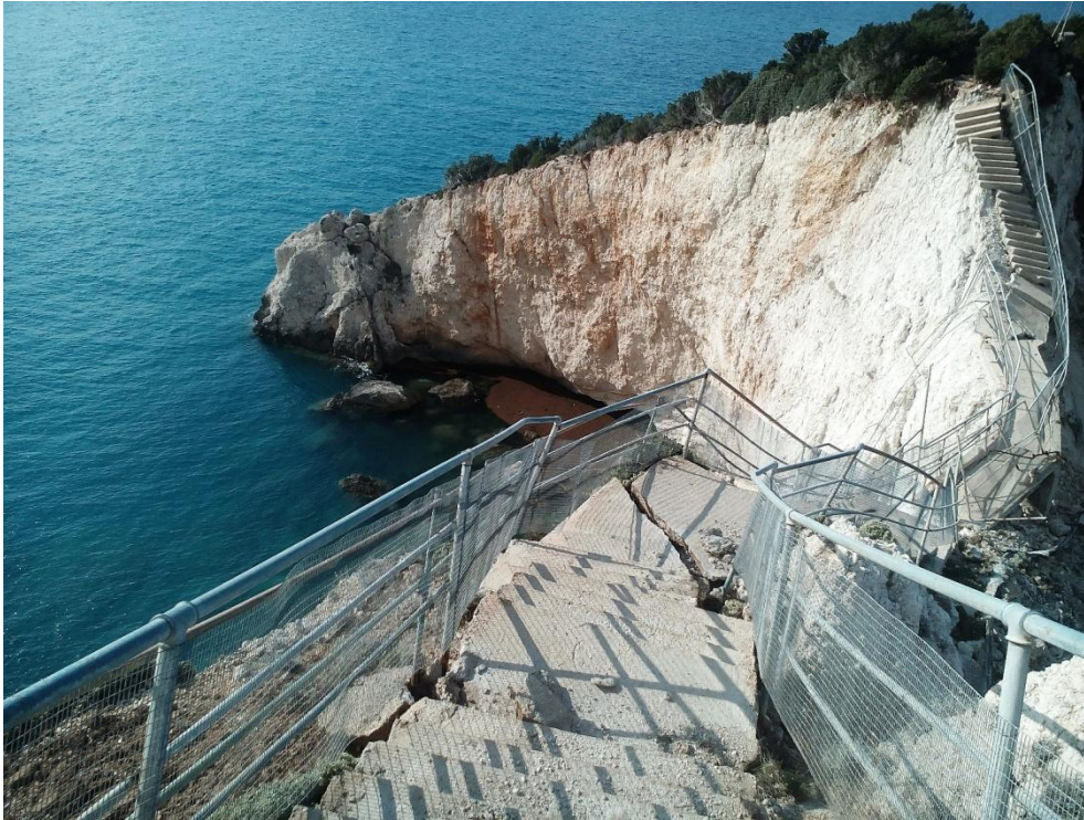
Figure A3 Field photo of damaged path to Porto Katsiki cape. View to the west. Date photo was taken 20 Nov. 2015.
